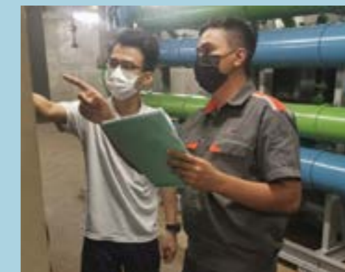
Mr Ahmad Syahir, Senior Assistant Engineer, SBS Transit conducts regular checks of the Water-Cooled Chillers at MRT stations, to ensure the desired temperature level at the stations is maintained.
